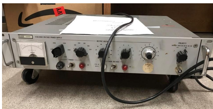
Fig. 3. High Voltage power supply system at GL
